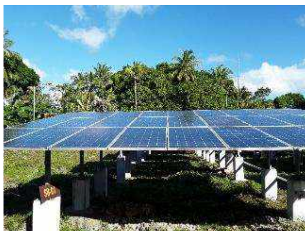
Figure 24: The broken PLTS at Pulau Tiga
