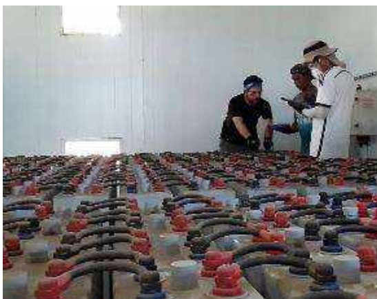
Figure 15: NZMATES technical team testing batteries on the PLTS in Lirang
