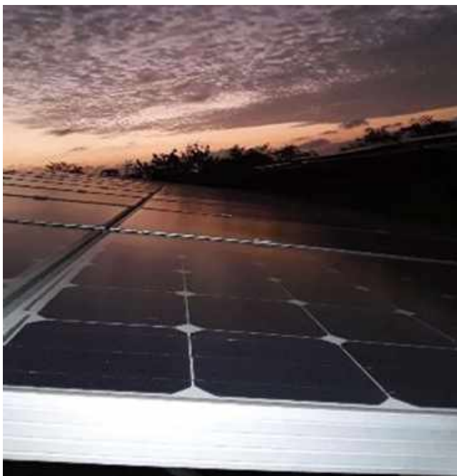
Figure 27: Sunset over the PLTS at Adaut.
