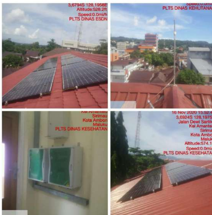
Figure 9: EBTKE Solar PV Rooftop Installations
