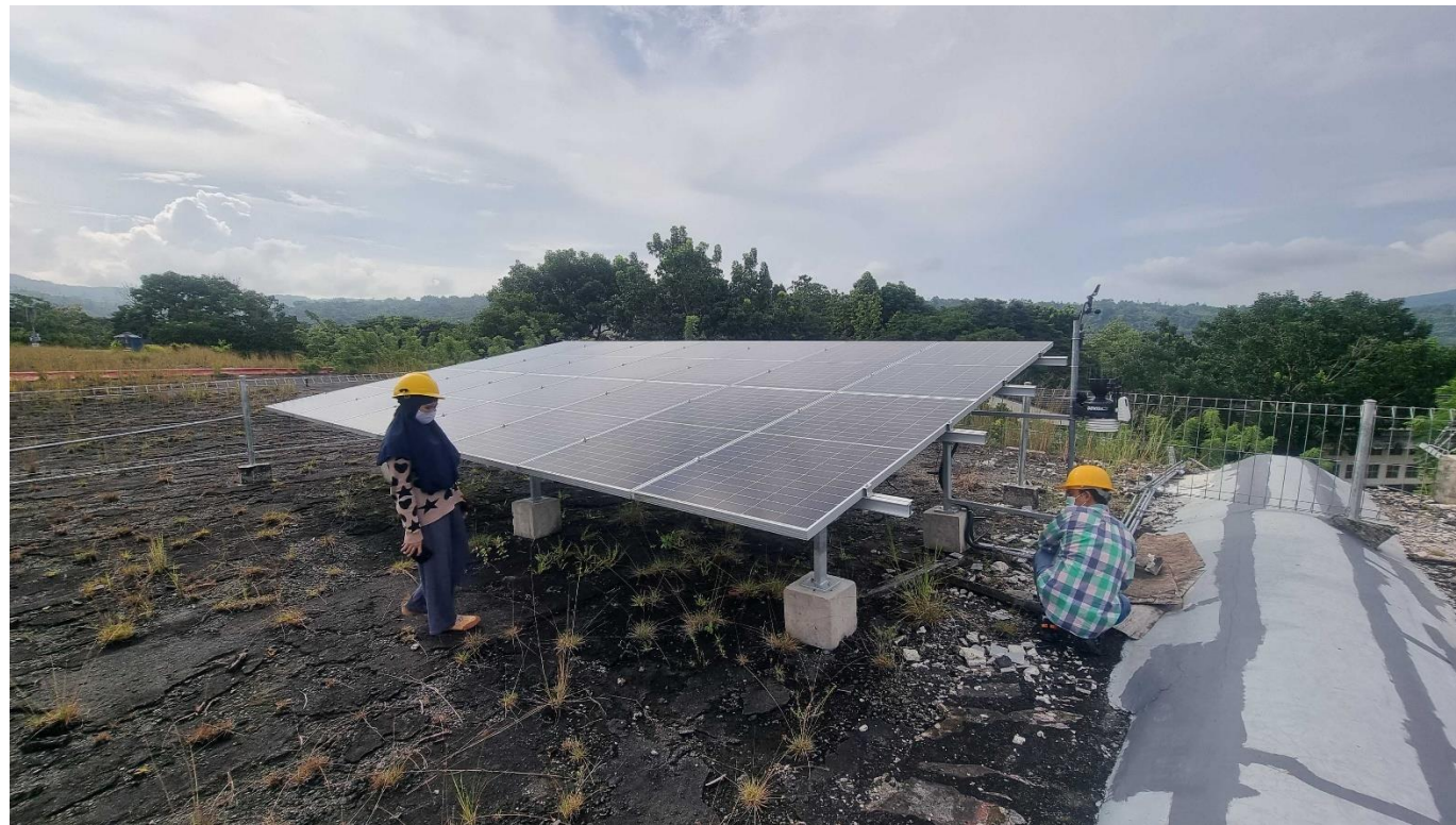
Figure 22: RETS Usep Nuraen and REJE Putri Hatuina carry out checks on the UnPatti solar lab PLTS.
