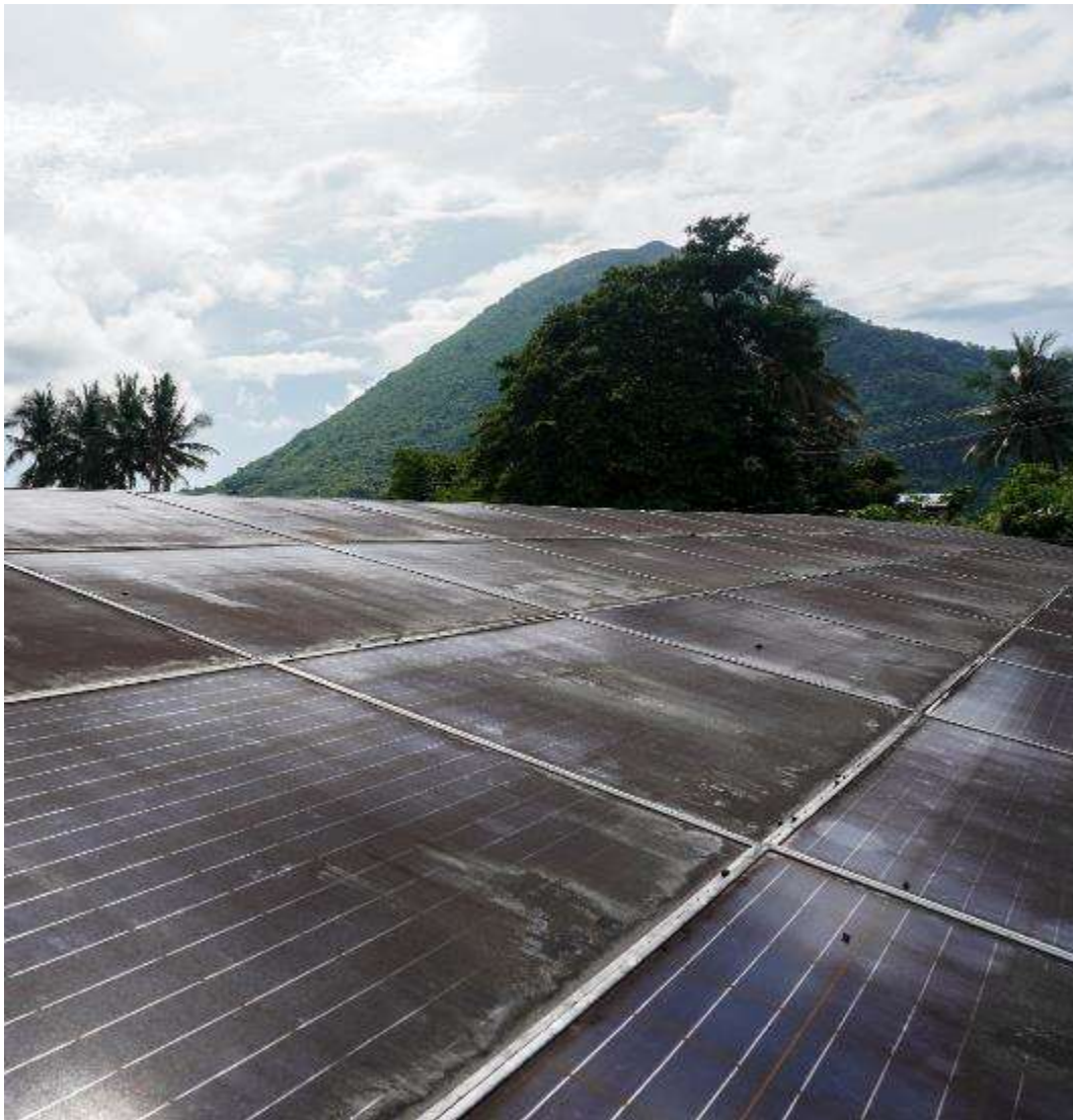
Figure 18: Broken PLTS surveyed for refurbishment on Banda Neira island. Old components, like the damaged panels seen here, need to be disposed of responsibly.
