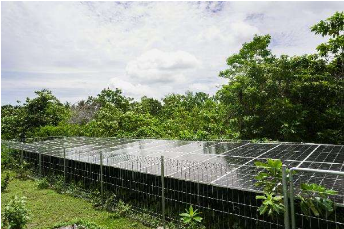
Figure 11: 17.2kWp PLTS installed at the Health Centre in the community of Dullah Laut.
